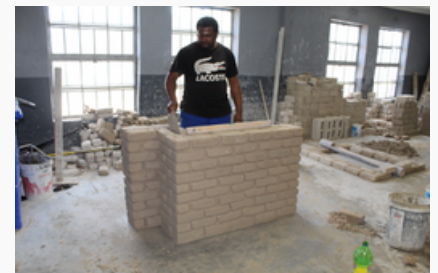
Above: The bricklaying team continues with its work, targeting unskilled individuals within the community and providing them with skills in hope that they will become self-sustaining.
